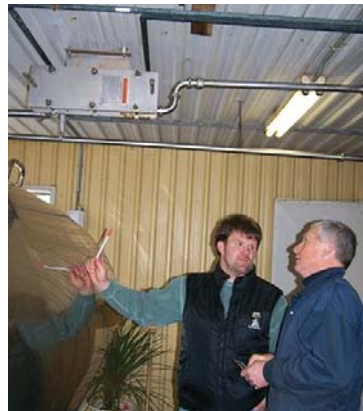
Terence Rothwell (right), project manager for OPA agriculture program design, and Korb Whale of Clovermead Farms, discuss the energy efficiency of the plate heat exchanger (shown in the upper left section of the photo), used for precooling the milk with cool well water before it enters the 10,000 litre milk tank.
